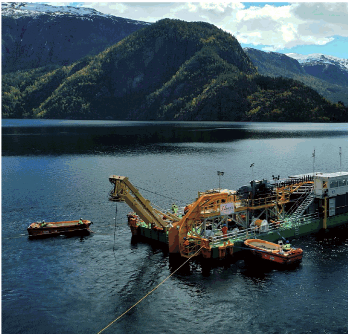
Construction of the North Sea Link, an interconnector between Norway and the UK, included building a custom barge
